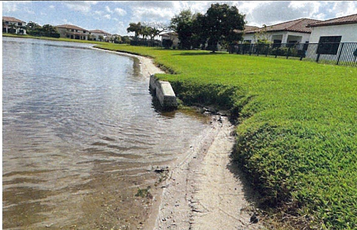
Photo 12: Lake 3 erosion by headwall
