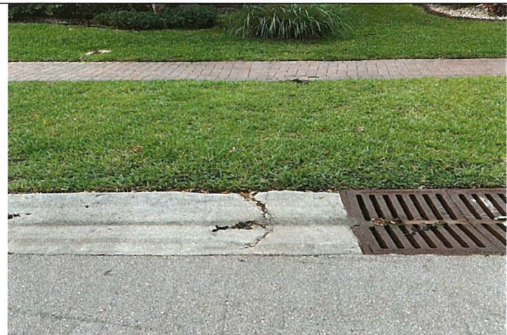
Photo 15: Broken curb 6380 Grebe Ct
