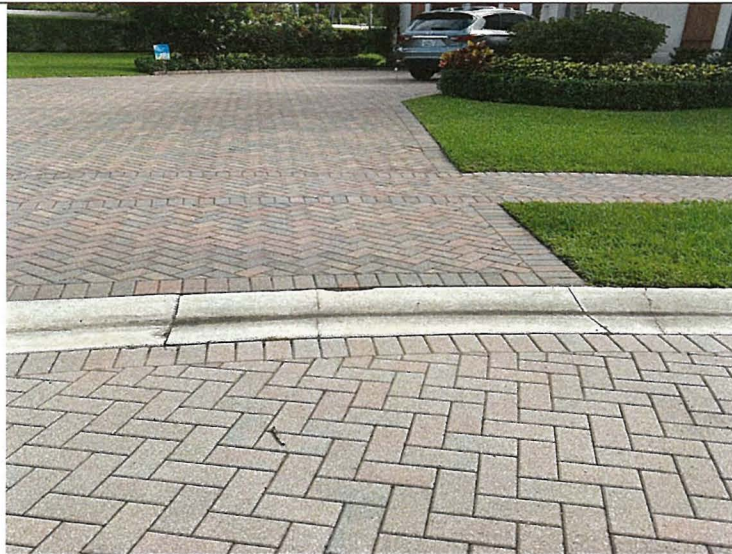
Photo 13: Broken curb 7030 Muscovy Ct
