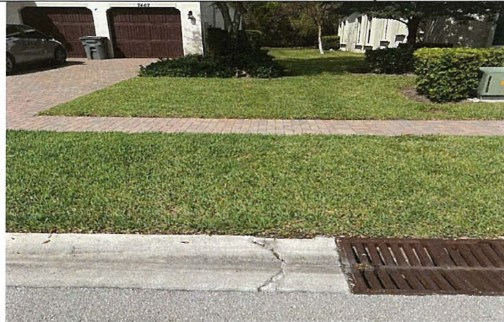
Photo 14: Broken curb 7467 Pochard Ct
